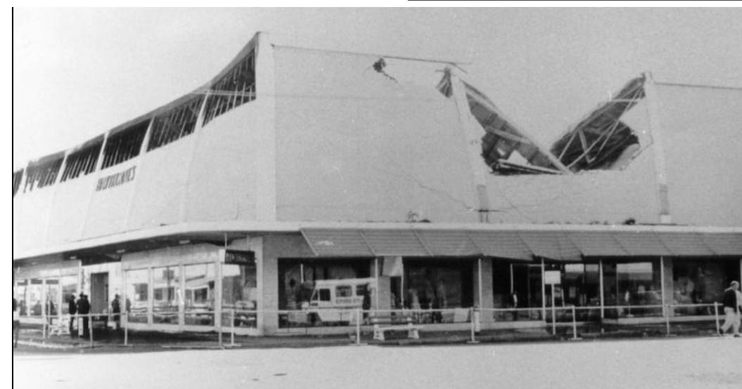
Below: Damage to the upper level is obvious from this photograph. Hydraulic platforms were engaged from the S.E.C. to assist the firefight.
