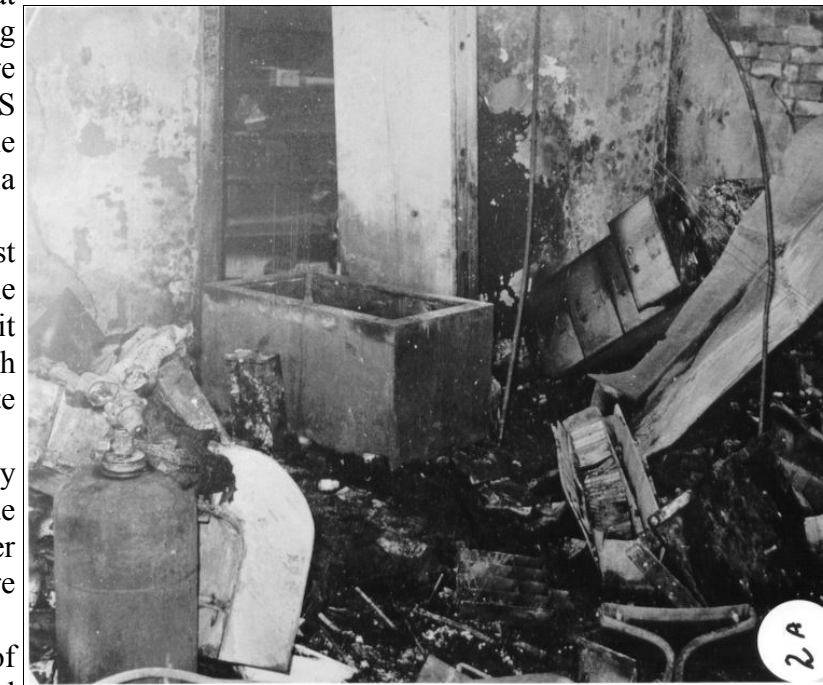
Above: The fire commenced in the vicinity of the Strong Room in the General Office. Note the cutting gear in the left of the photograph.
