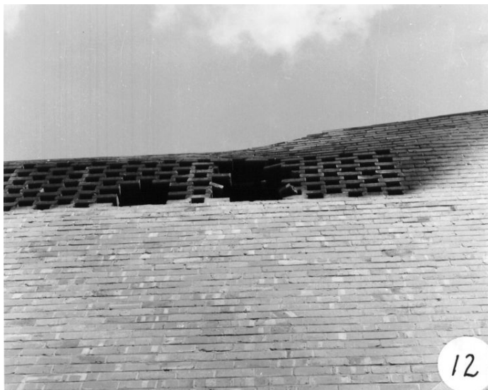
Above;- The lattice brickwork over the 1st floor toilet windows taken from ground level in the narrow side lane.
